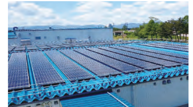
Solar panels at Kitakami
